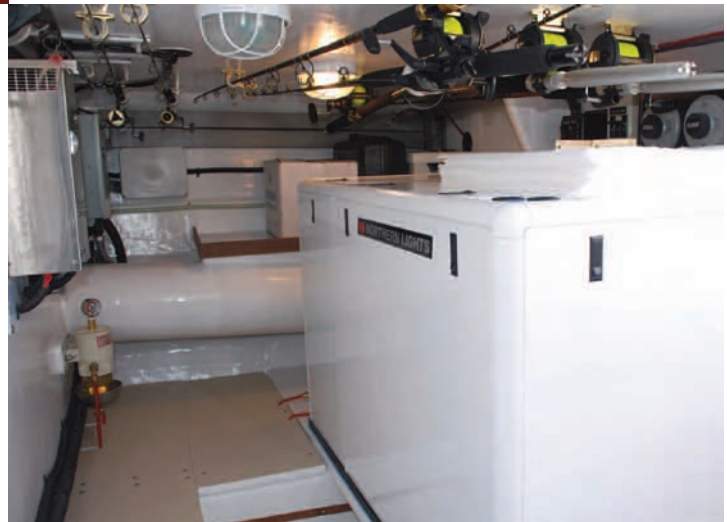
Above left: Upgraded to 853hp Cat C15s, Island Bird has an engine room with exceptional access to all sides of the engines and systems. Above: A separate compartment aft holds the twin Northern Lights generators and electrical systems, plus storage for cruising gear.
